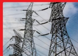
Wind power nuclear power UHV
